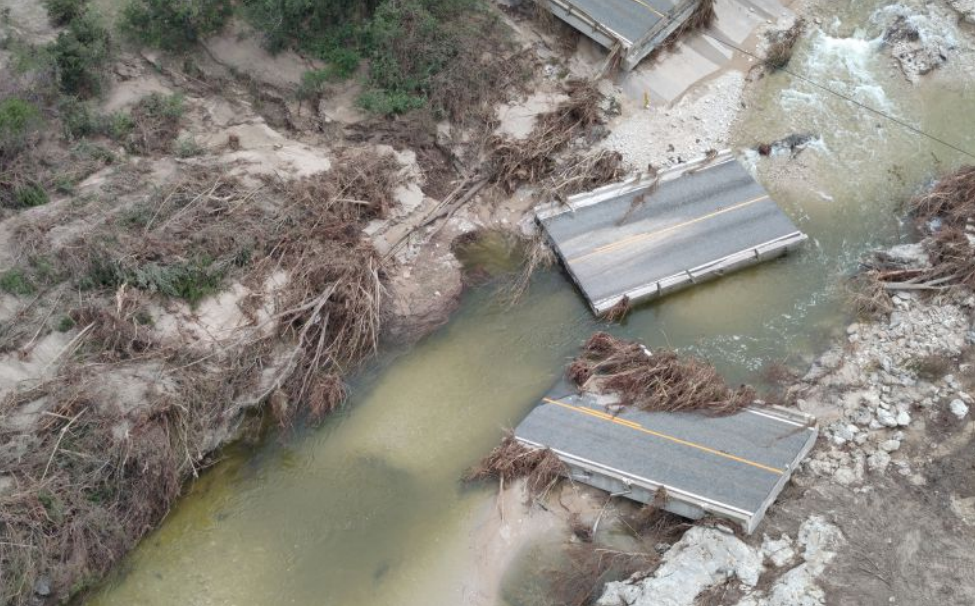
The original bridge was overtopped by Cow Creek, and segments were displaced some distance away. All Photos: Texas Department of Transportation.
