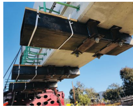
View from beneath an edge girder. No falsework was permitted in the creek, so the team developed a temporary support system to support the floor beams during construction. The supports were later repurposed to facilitate installation of the bridge's transverse post-tensioning. All Photos: Stacy Witbeck/Herzog.
