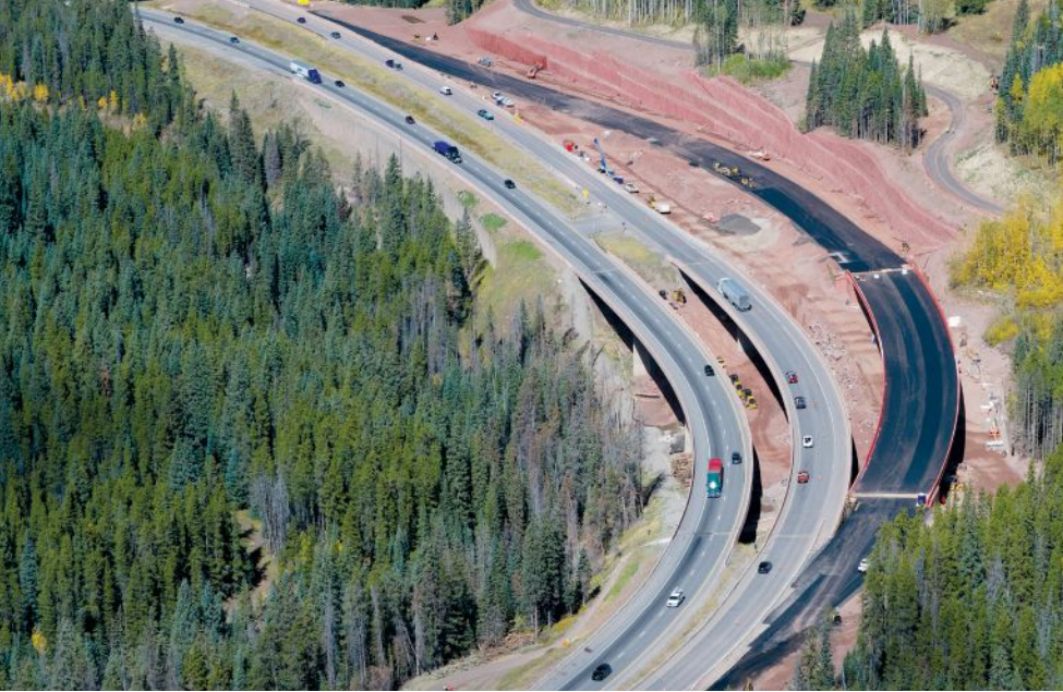
The difference in width and curvature between the original Interstate 70 (I-70) over Polk Creek bridges (left) and the nearly completed westbound bridge (right) is clear in this photo. By widening traffic lanes and shoulders and modifying existing curves to meet current federal design standards, the project improves safety and operations on I-70 for the traveling public. Photo: Dennis Humphrey, Cirque Civil.
