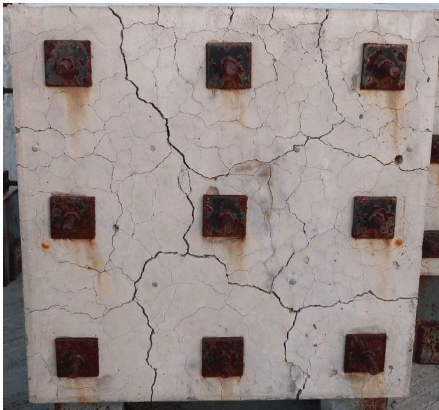
Figure 1. Cracking related to alkali-silica reaction (ASR) in a cube that is reinforced in one direction (into the page). The specimen was cast in 2015, and the photo was taken in 2023 as part of long-term monitoring of ASR-affected reinforced concrete cubes. Photo: Concrete Bridge Engineering Institute.
