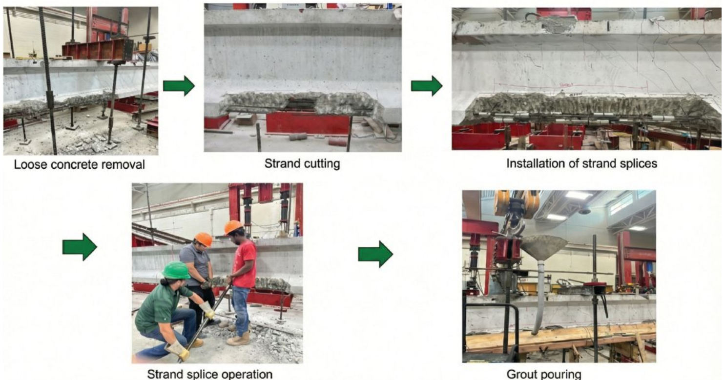
Figure 6. After the girders were impact tested, these steps were taken in the strand splicing repair.
