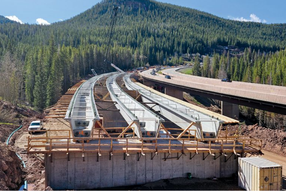
Temporary diaphragms were installed between girders to prevent girder distortion during deck placement and ensure stability. The bridge engineer designed temporary diaphragms at midspan (steel K-frames in this photo). The contractor designed temporary diaphragms at girder ends (wood timber and steel rods in this photo). Photo: Kevin Petrillo, RockSol.
