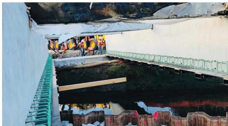
Timber struts provide bracing to mitigate the inward rotation of the edge girders during installation of the floor beams. After each floor beam is set, the shims at the strut ends are adjusted.
