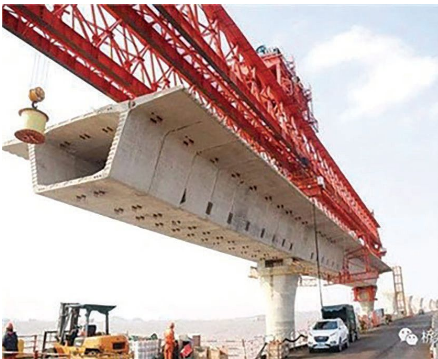
Figure 1. A concrete segmental bridge structure is constructed using precast concrete segments. Figure: Datai Crane.
