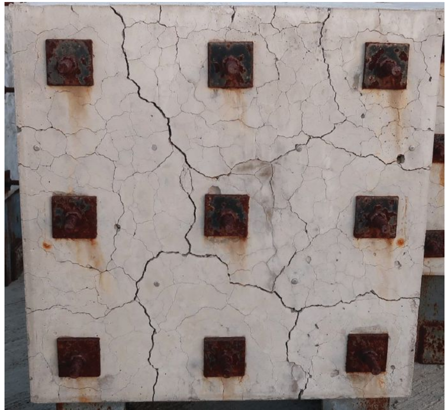
Figure 1. Cracking related to alkali-silica reaction (ASR) in a cube that is reinforced in one direction (into the page). The specimen was cast in 2015, and the photo was taken in 2023 as part of long-term monitoring of ASR-affected reinforced concrete cubes. Photo: Concrete Bridge Engineering Institute.
