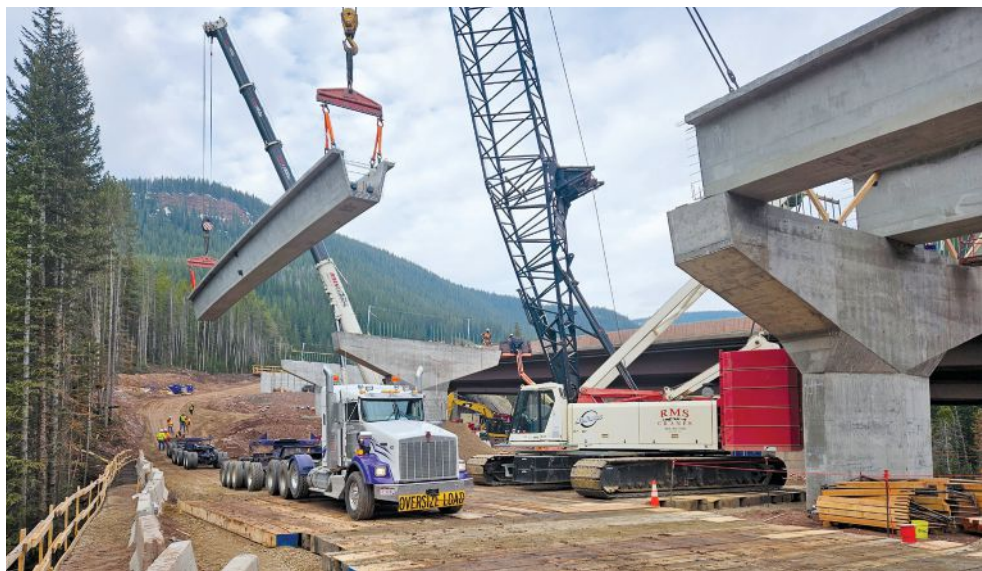
One of the precast concrete tub girders for span 3 of the westbound structure—with a girder weight of approximately 220,800 lb—is lifted to its final position on the piers. The simple-made-continuous for live-load concept for the Interstate 70 over Polk Creek bridges saved considerable time by eliminating the need for falsework towers. Photo: Kevin Petrillo, RockSol.
