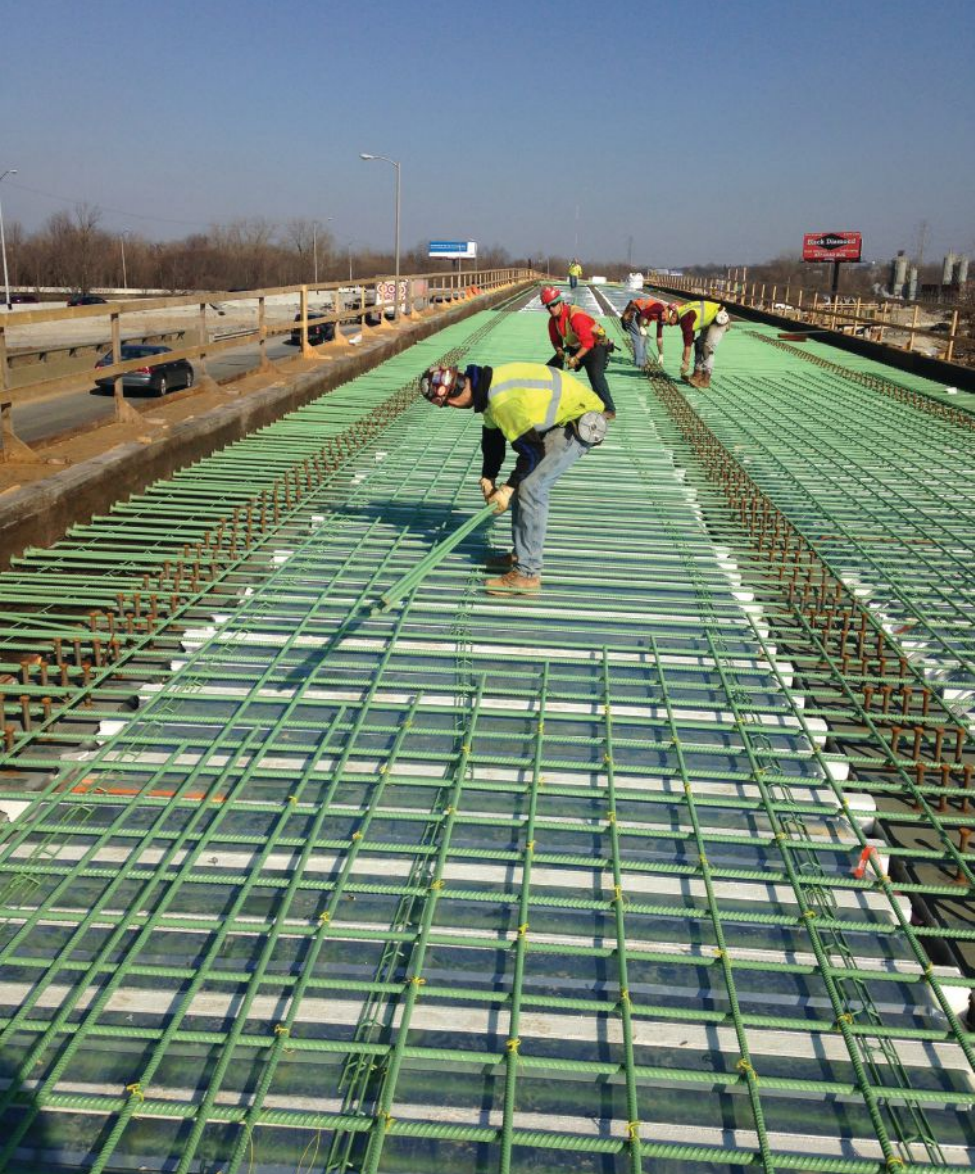
Workers place epoxy-coated reinforcing steel for a bridge deck, with bars supported at the specified elevation to maintain concrete cover during concrete placement.
