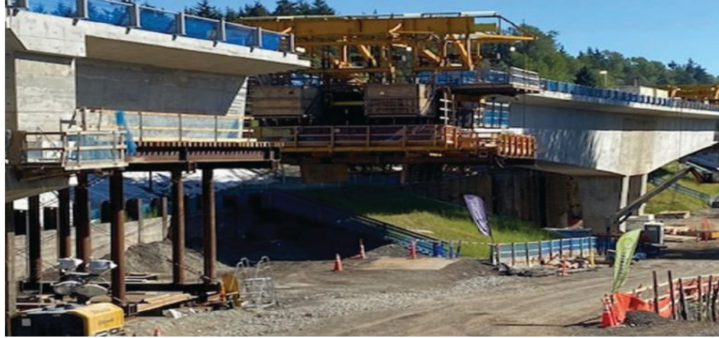
Two sections of the back spans were cast on falsework at either end of the structure for a length of about 50 ft, while the remainder of the segmental structure was constructed using form travelers and the balanced-cantilever construction method. Photo: Kiewit.
