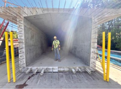
Cast-in-place concrete box-girder segments vary in height from 12.5 ft at the midspan to 25 ft at the piers and typically have a width of 28 ft 9 in. The bottom-slab post-tensioning ducts and web shear keys are visible. Photo: Kiewit.
