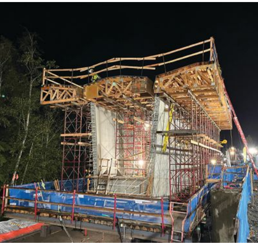
Integrated shop drawings and three-dimensional modeling allowed the design team to spot conflicts before they happened, which was critical to the successful installation of the many reinforcing elements required in the superstructure. Photo: Kiewit.
