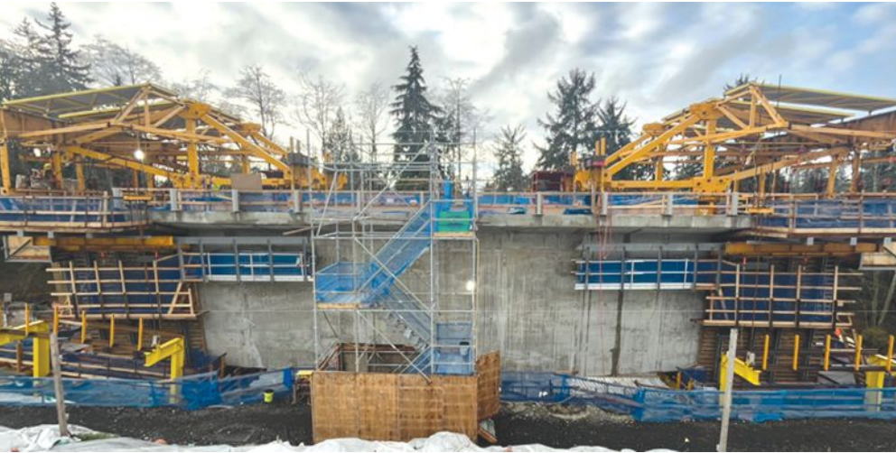
Segments are being cast on both sides of one of the piers. Using four identical form travelers allowed segments to be cast on both sides of both cantilevers concurrently. Photo: Kiewit.
