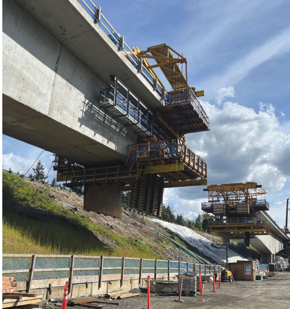
Structure C was completed in October 2024 and Sound Transit plans to begin systems integration testing along the extension as early as the end of 2024. Photo: Kiewit.
