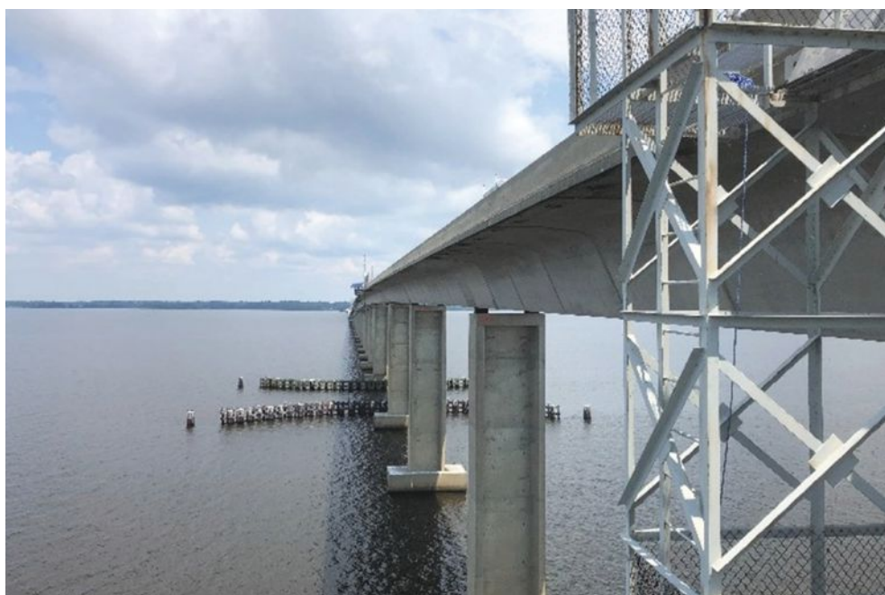
Siva Corrosion Services performs a corrosion evaluation of internal tendons in the trestle spans and external tendons in the concrete segmental box girders along the 18,460-ft-long Albemarle Sound Bridge. All Photos: Siva Corrosion Services.
