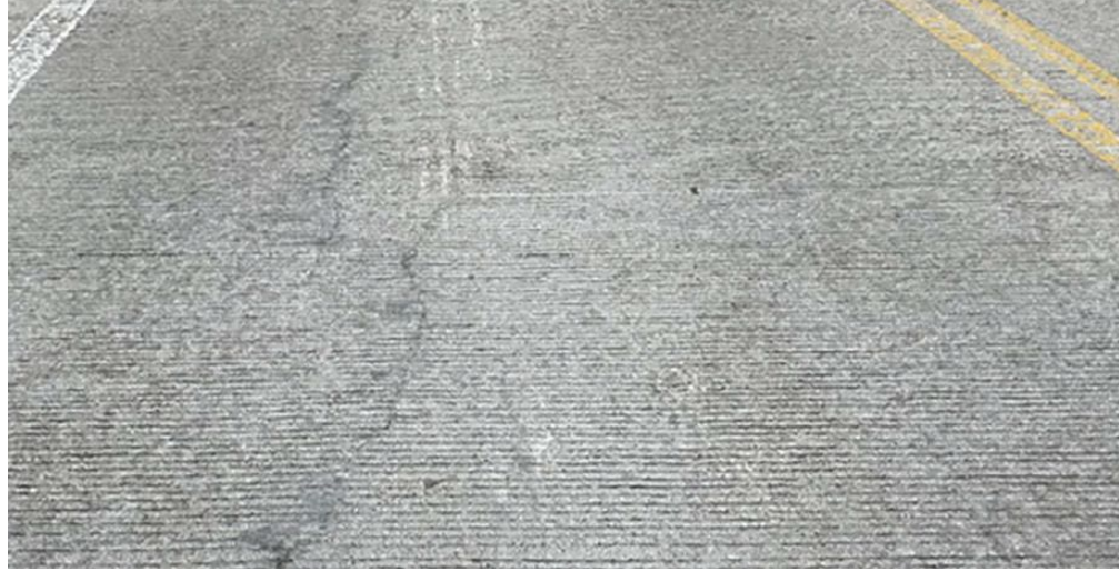
An example of longitudinal cracking in a concrete bridge deck.
