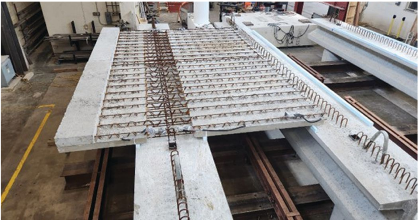
The Concrete Bridge Deck Inspection Site will have a location for new bridge technologies, including the NextGen Deck Panels. Photo: Concrete Bridge Engineering Institute.
