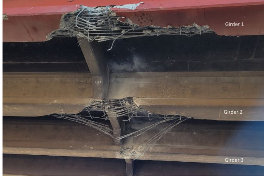
Figure 8. In October 2022, the NM 129 overpass over Interstate 40 was hit by an excavator and all strands were severed on two of the five prestressed concrete girders. One lane was immediately closed and remains closed. Construction to replace the damaged span is anticipated to begin in late 2024. Photo: New Mexico Department of Transportation.
