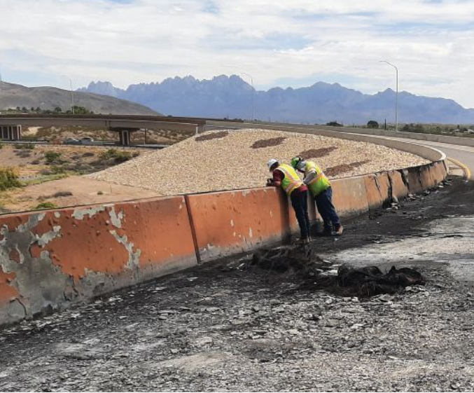
Figure 7. In July 2023, a fuel tanker truck overturned and burned, resulting in fire damage to a concrete bridge deck and barriers. The fire-damaged concrete was repaired or removed and replaced. The structure was reopened five months later. Photo: New Mexico Department of Transportation.
