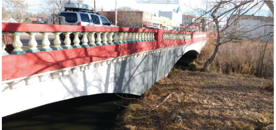
Figure 1. New Mexico's oldest concrete arch bridge carries Bridge Street over the Gallinas River in Las Vegas, N.Mex. It was built in 1909 and is still in service today. Photo: New Mexico Department of Transportation.
