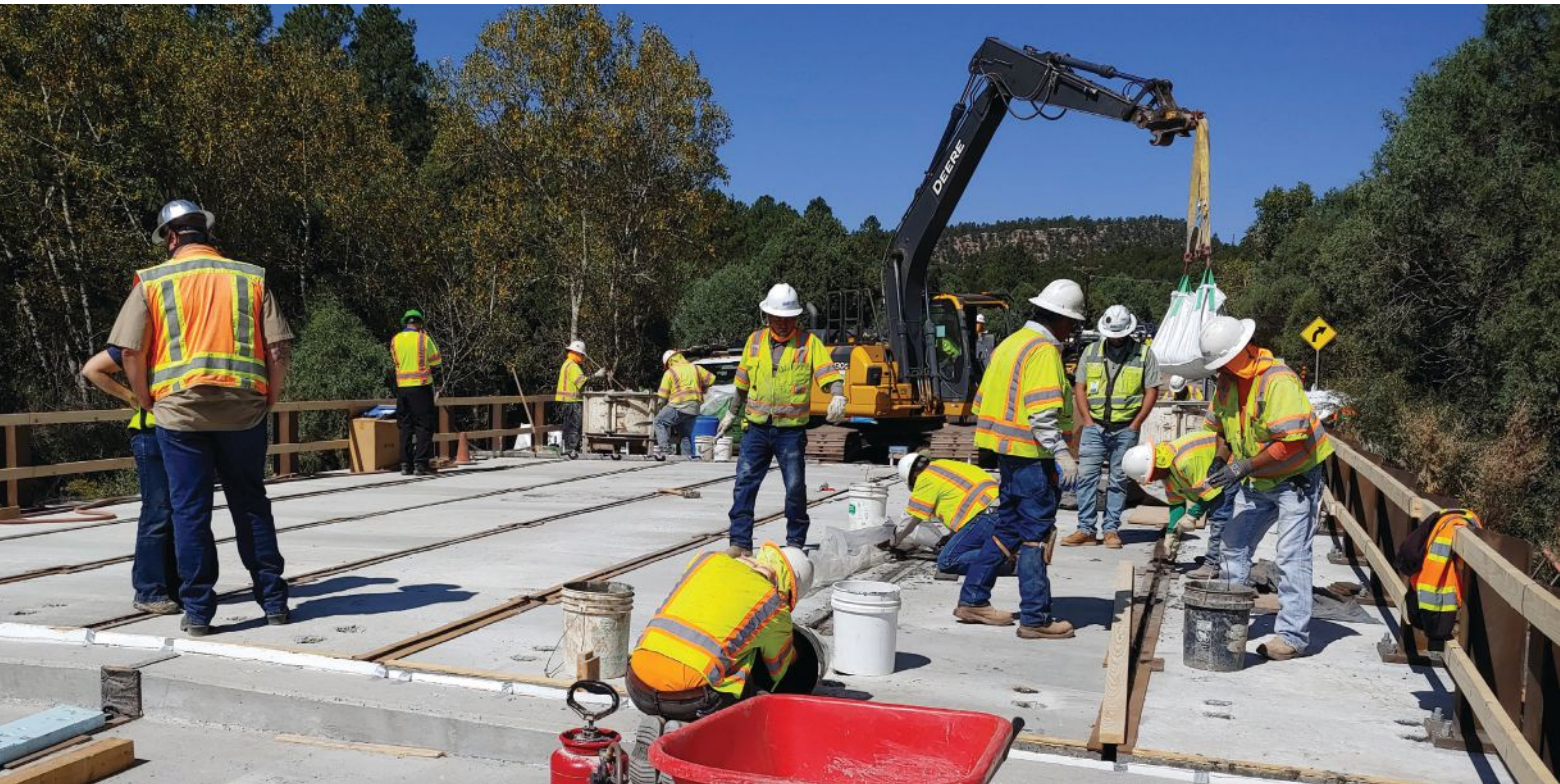
Figure 6. Installation of ultra-high-performance concrete joints on the NM 50 over Glorieta Creek Bridge. Photo: New Mexico Department of Transportation.
