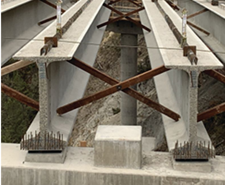
Figure 4. Typical wood cross bracing helps distribute wind load to all girders but does not provide additional strength to individual girders. Photo: Kicking Horse Canyon Constructors.
