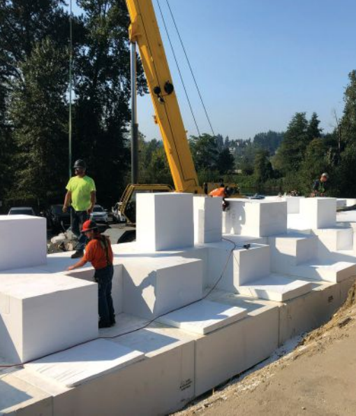
At the roadway approaches, geofabric blocks are placed over traditional gravel materials to mitigate settlement of the highly compressible peat layers. Photo: City of Kenmore.
