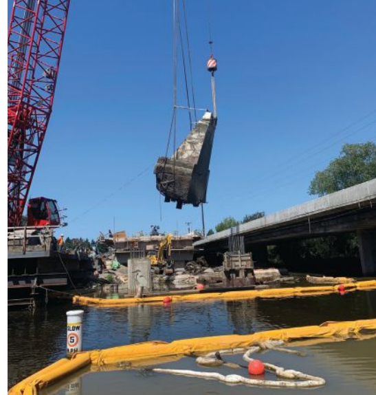
In two cases, removal of the existing concrete foundation required that sections be cut in half. Photo: City of Kenmore.
