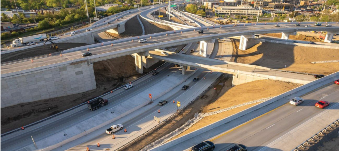
Aerial view of the North Split Project north of downtown Indianapolis, Ind., where Interstates 70 and 65, including local access and exit ramps, intermingle. Photo: Indiana Department of Transportation.
