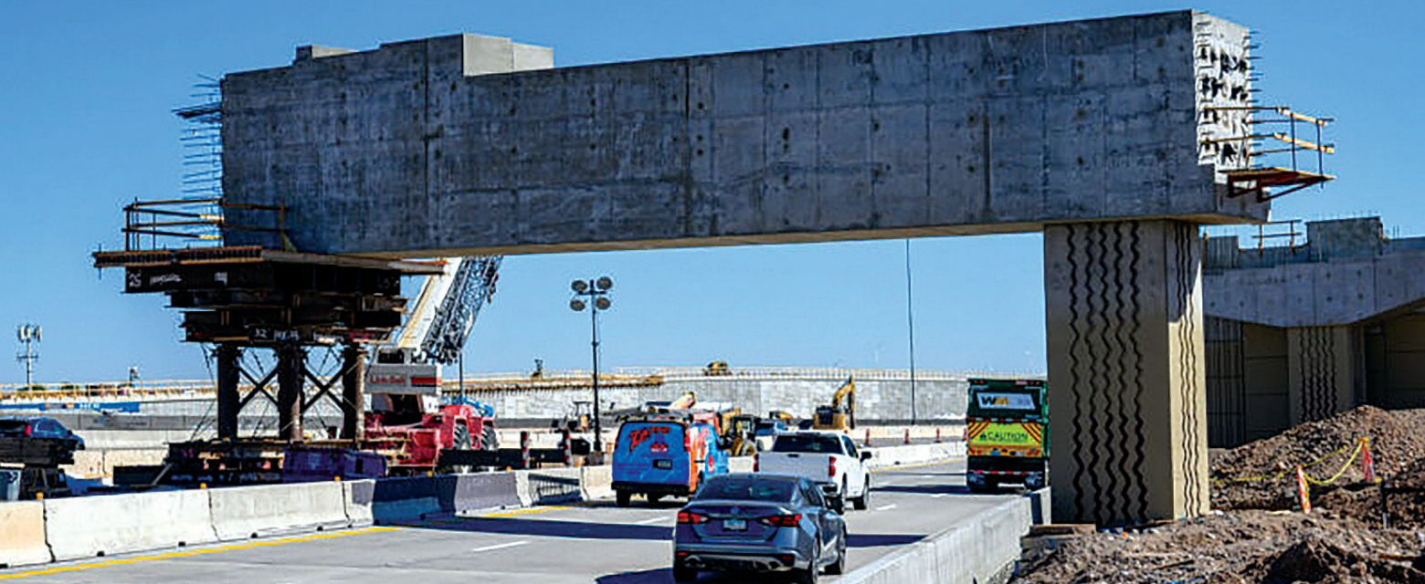
In March 2024, workers constructed the concrete straddle bent in the Interstate 10 median work zone between Broadway Road and State Route 143. The structure will carry ramps connecting high-occupancy vehicle traffic between I-10 and SR 143. Photo: Arizona Department of Transportation.
