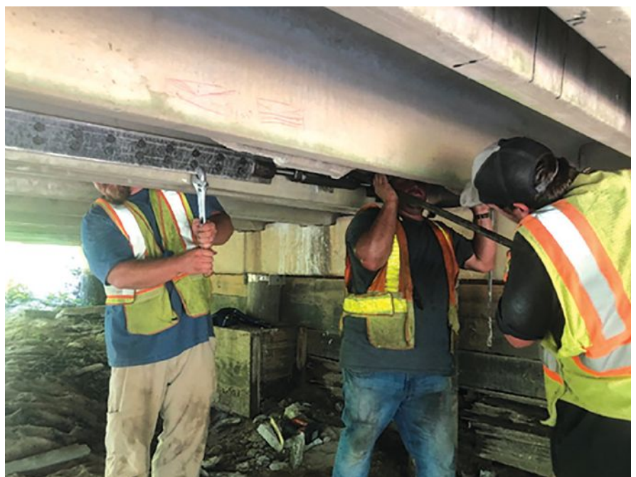
Figure 3. A North Carolina Department of Transportation maintenance crew prestresses a fiber-reinforced-polymer plate by tightening a turnbuckle on the Sampson County bridge.
