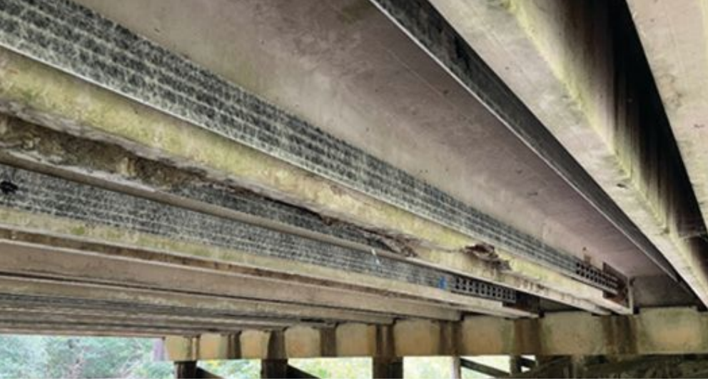
Figure 4. Completed installation of the repair system before the reopening of the Sampson County bridge in November 2020.
