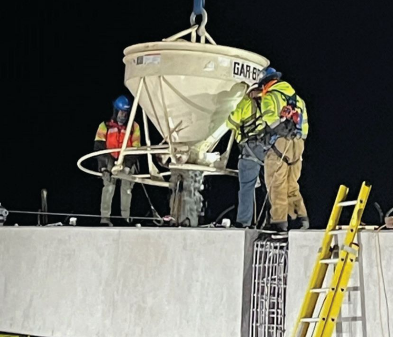
Concrete is placed for the connection between the 54-in.-diameter cylinder pile and a precast concrete bent-cap segment. The stainless steel reinforcement in the bent-cap closure joint is visible. Photo: Hampton Roads Connector Partners.
