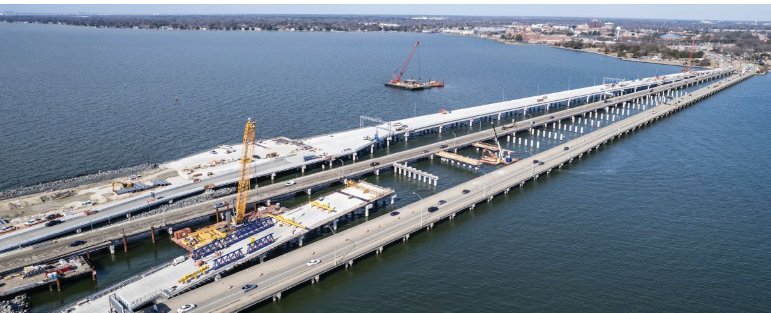
The new north trestle is constructed as two separate four-lane structures. Photo: Virginia Department of Transportation.
