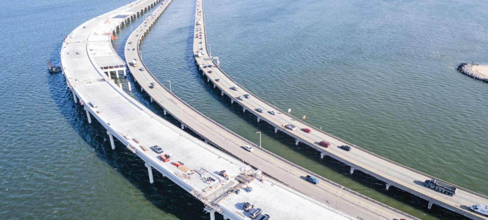
The new eight-lane south trestle is constructed in phases to maintain traffic on the existing trestles. Photo: Virginia Department of Transportation.
