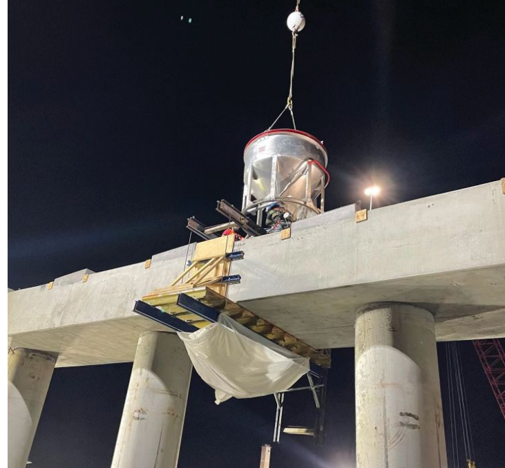
Concrete is placed at a closure pour between two precast concrete bent-cap segments. The design-build team used the alternative technical concept of precast concrete bent-cap segments spliced in the field to facilitate staged construction. Photo: Hampton Roads Connector Partners.
