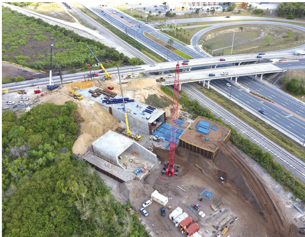
Figure 1. Precast concrete boxes are jacked horizontally into place under State Route 528 for the Brightline high-speed rail underpass in Cocoa, Fla. Photo: Granite Construction.
