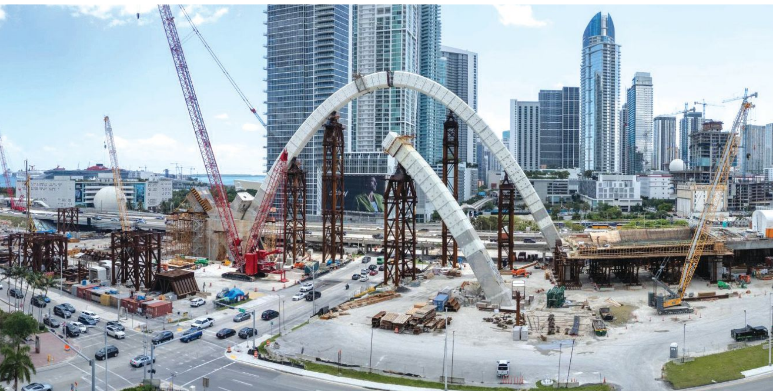
Figure 4. Arch No. 2 approaching keystone closure as part of the Interstate 395 Signature Bridge project in Miami, Fla. Unique structures require extensive construction engineering services. Photo: Archer Western.
