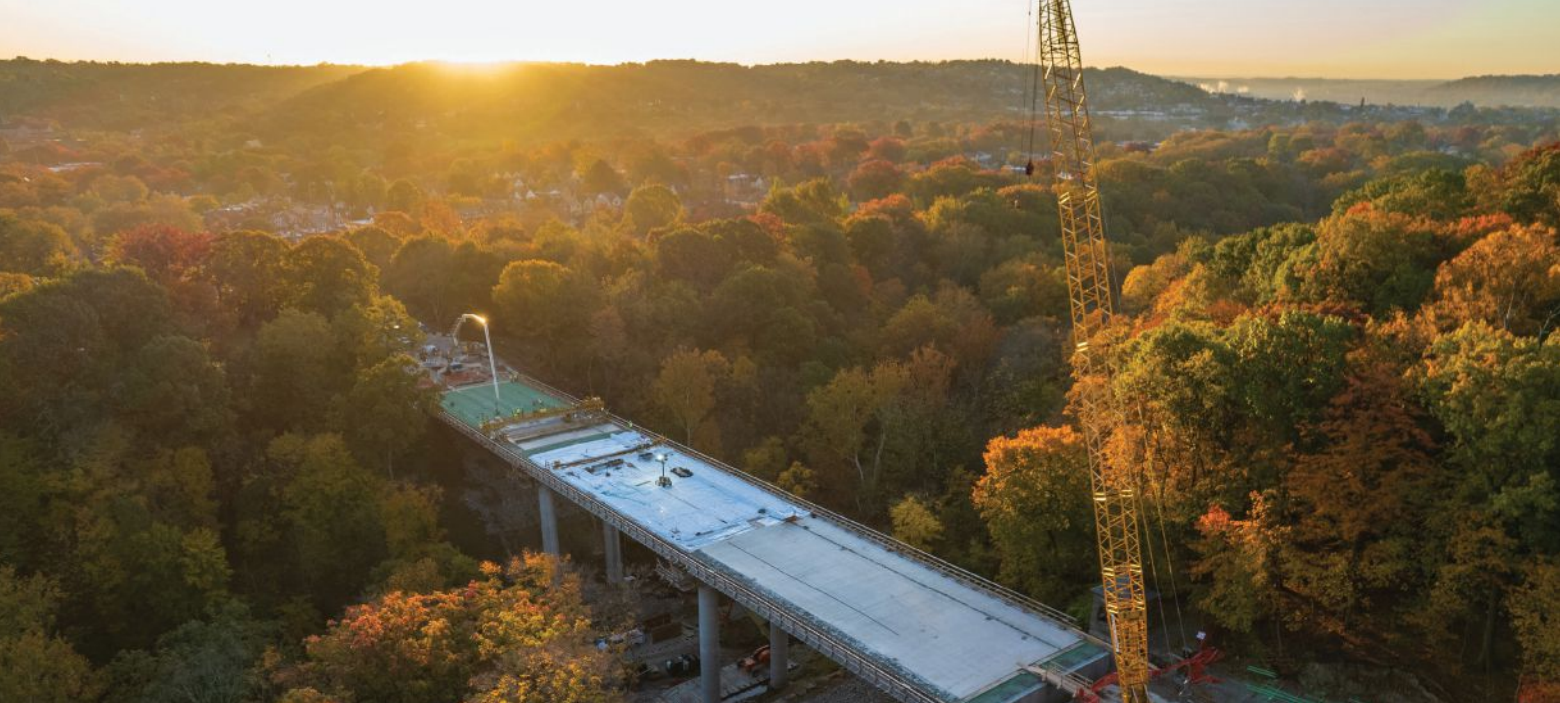
East-southeast view of concrete deck work continuing on the east side (span 3) of the new Fern Hollow Bridge in Pittsburgh, Pa., in October 2022. Photo: Swank Construction Co.
