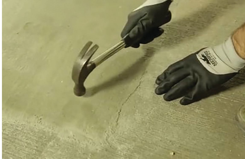
Figure 2. Identifying delaminated concrete using a sounding technique.
