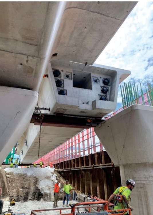
A pocket-track girder slides laterally into position. The post-tensioning hardware is visible in the box girder. Photo: Walsh-Fluor Design-Build Team.
