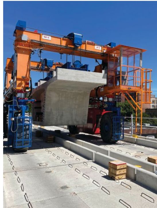
A rubber-tired segment transporter delivers a segment to the launching girder. Photo: Walsh-Fluor Design-Build Team.
