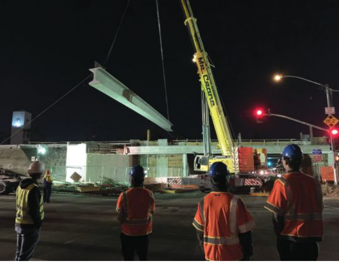
San Diego State University students get a close-up view of California wide-flange girder erection on Interstate 10 in Ontario, Calif. Photo: Con-Fab California.
