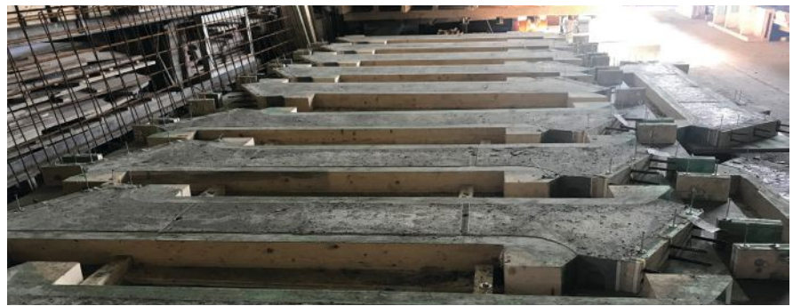
Struts are in their formwork at the precast concrete plant. Four types of forms were required. Photo: IngPhi SA, Lausanne.
