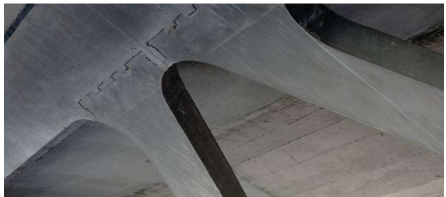
The completed connection of the prefabricated strut to the cast-in-place upper chord shows the adjustability to the geometry that the innovative construction detail allowed. Photo: IngPhi SA, Lausanne.
