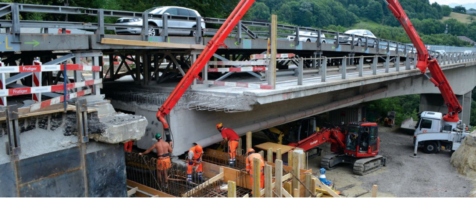
The Swiss Federal Roads Office's temporary steel bridge (flyover) on the deck of the bridge resulted in a 12-ft-long work area across the entire width of the bridge that accommodated 40-mph traffic during construction activities. Photo: IngPhi SA, Lausanne.
