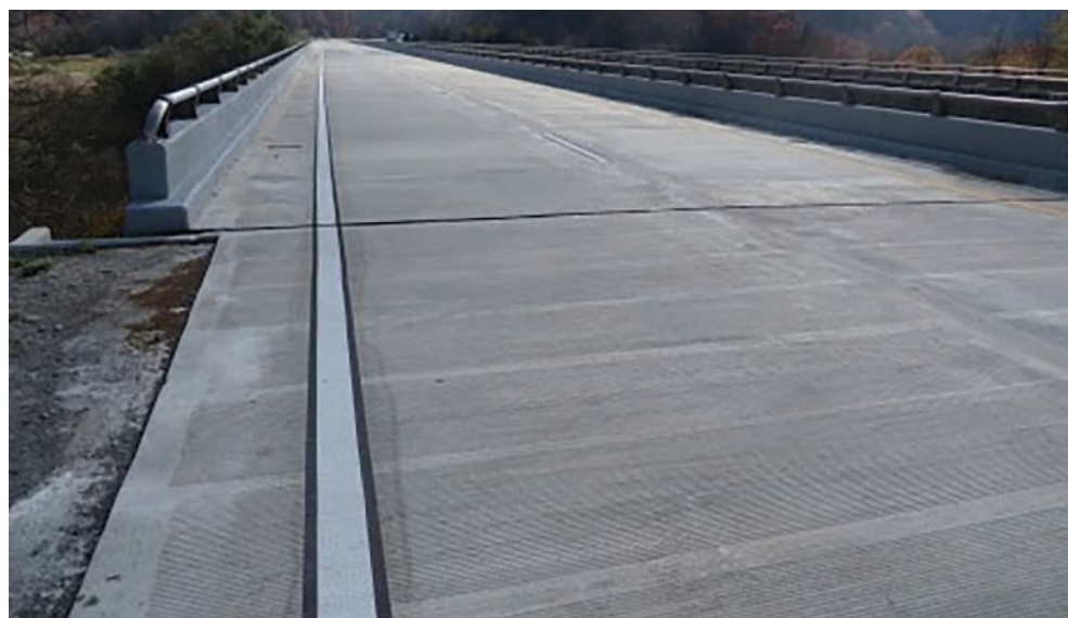
Figure 4. Preservation strategies for this Interstate 64 bridge included bearing reconfiguration to accommodate joint closures, deck extensions, hydromilling, and overlay replacement for a comprehensive jointless solution.
