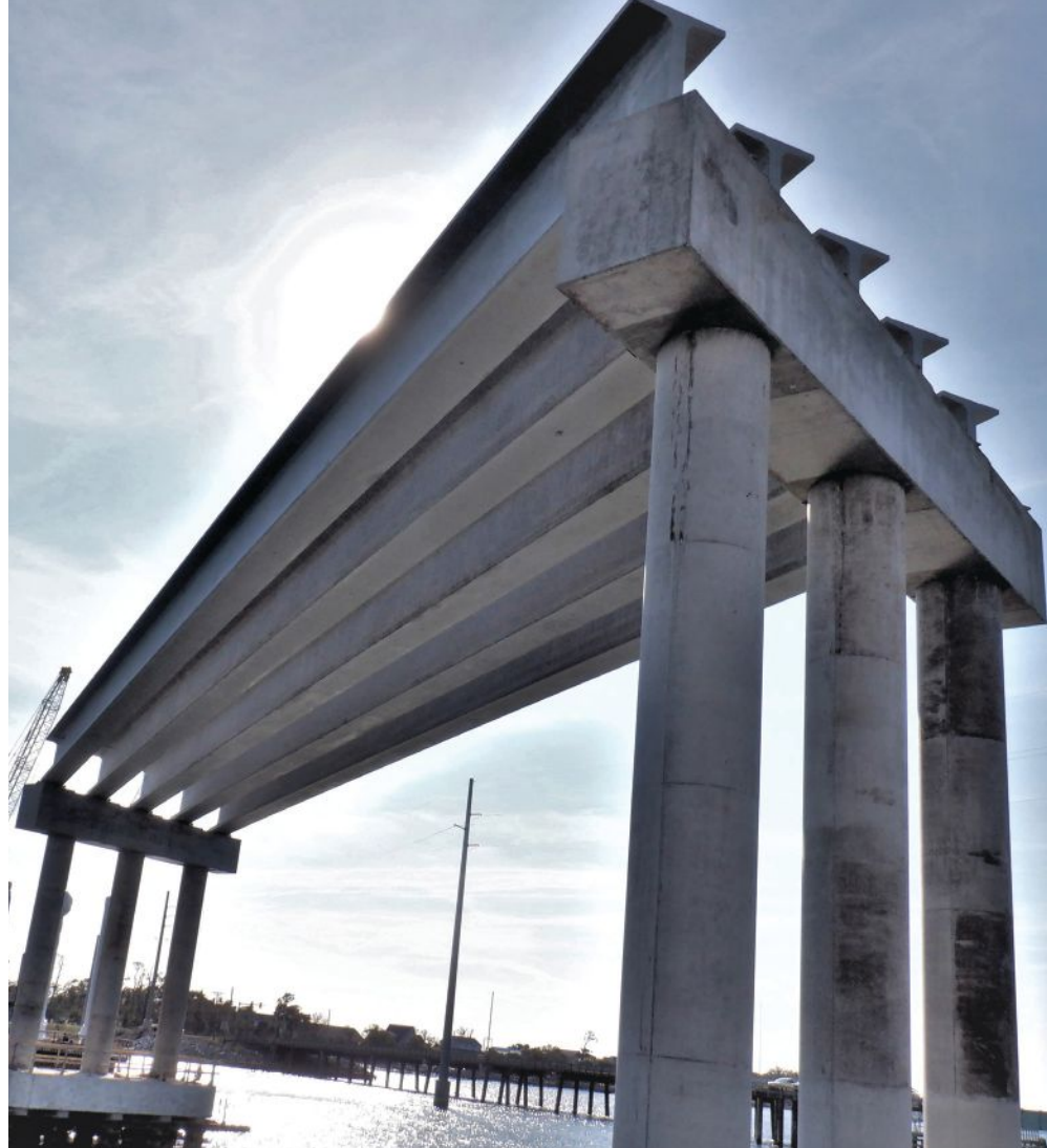
The 164-ft navigational span features five 78-in.-deep Florida I-beams with glass-fiber-reinforced-polymer stirrups and prestressed with carbon-fiber-reinforced-polymer strands. The span provides 125 ft of horizontal clearance and 45 ft of vertical clearance for vessel traffic. Photo: North Carolina Department of Transportation.
