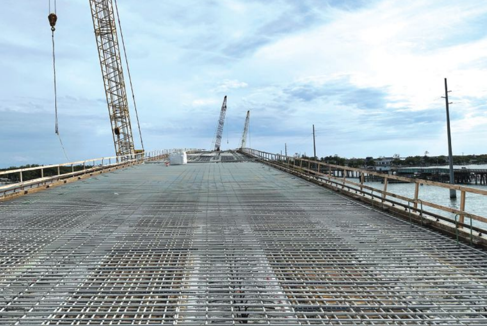
The 8¼-in. sand lightweight concrete deck is reinforced with no. 6 glass-fiber-reinforced-polymer bars. Removable forms are used for deck construction. Photo: North Carolina Department of Transportation.
