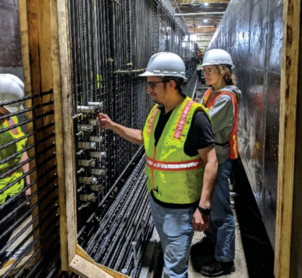
Before a Florida I-beam girder is cast at the plant, prestressed carbon-fiber-reinforced-polymer strands and glass-fiber-reinforced-polymer transverse reinforcement are placed. Students at North Carolina State University have the opportunity to participate in research projects associated with actual construction projects.
