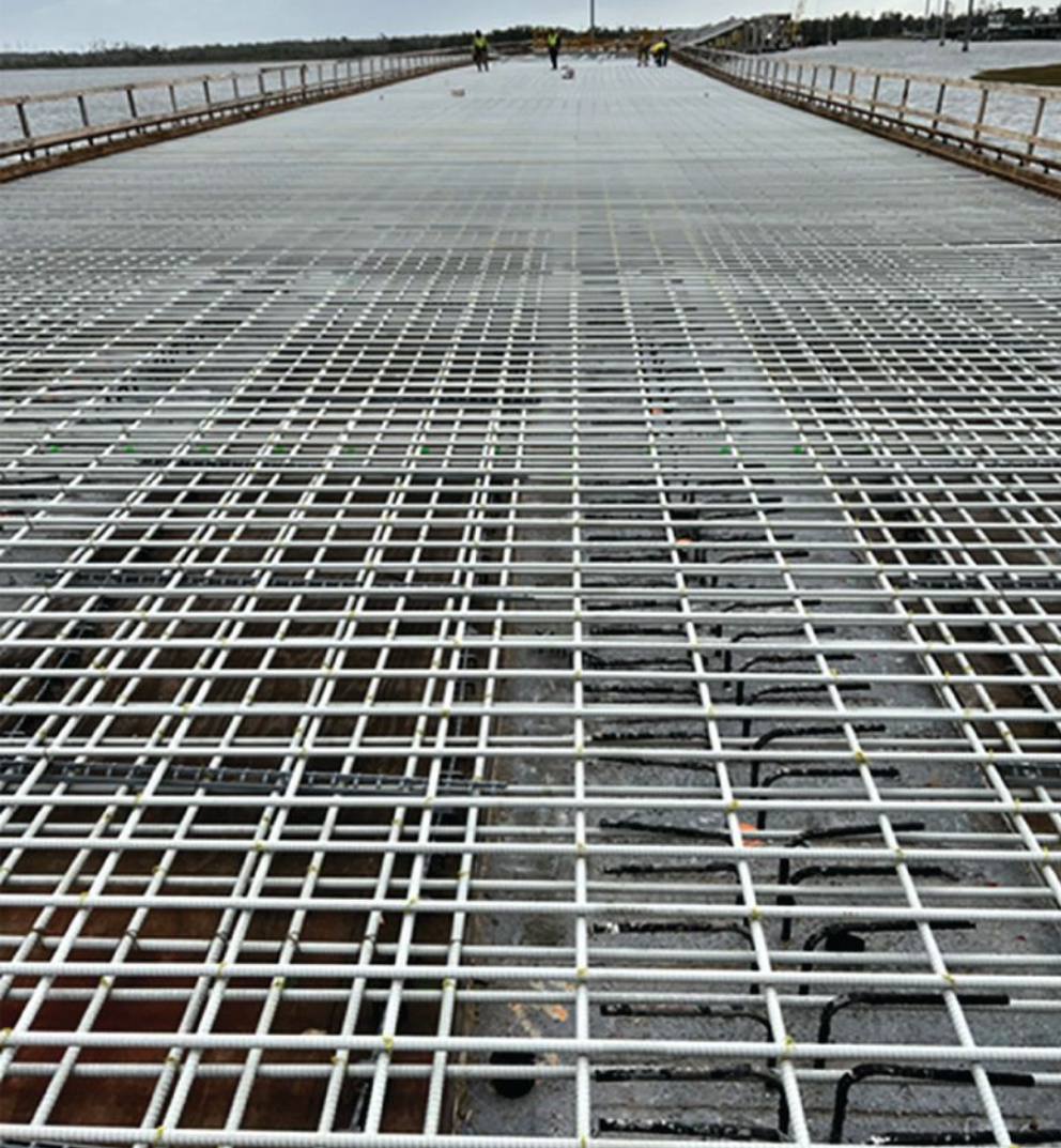
Glass-fiber-reinforced-polymer reinforcement was used in a cast-in-place concrete bridge deck and for the stirrups, which can be seen protruding from the prestressed concrete Florida I-beam girders.
