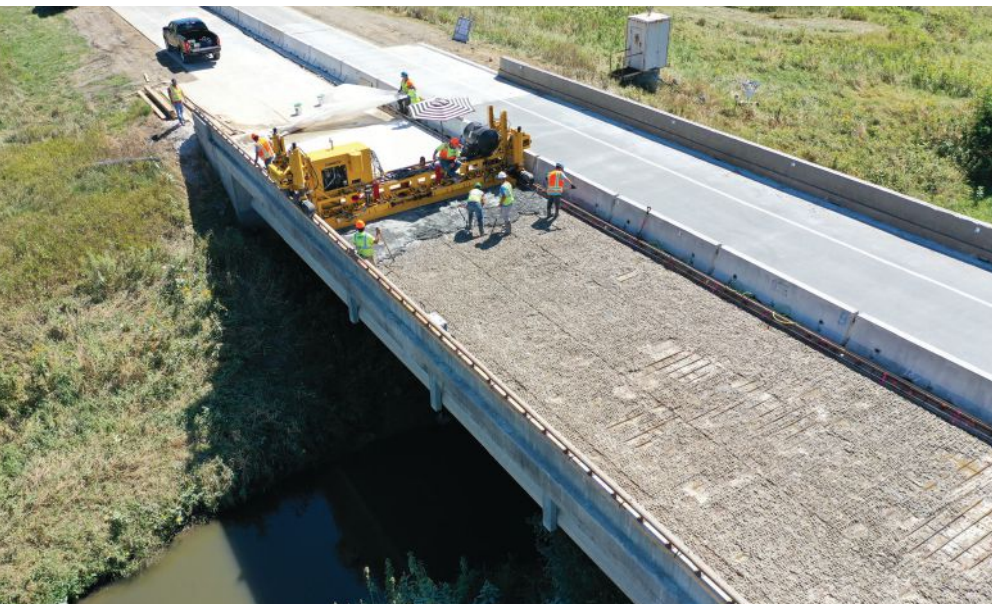
A drone-captured image of the ultra-high-performance concrete (UHPC) bridge deck overlay process in Jasper, Iowa. To extend the life of the existing bridge, a thin layer of UHPC was placed on the deck as a protective layer, sparing the expense of deck repair and full deck replacement. The Iowa Department of Transportation readily shares information on its use of UHPC in overlays.
