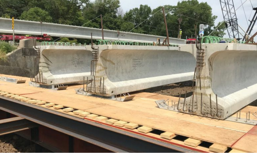
The precast, prestressed concrete beams for the Iowa Route 1 Bridge over Camp Creek are set on temporary falsework to construct the bridge superstructure off alignment. There are stainless steel slide shoes under the beams for the lateral slide of the new 120-ft-long, 44-ft-wide bridge.
