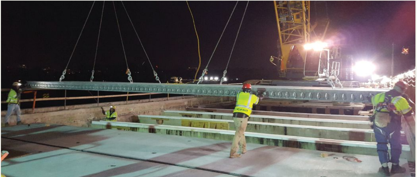
Precast concrete deck panels were installed at night, when traffic volumes were low. Panels span between the cross walls that are visible in the center of the photo. The bridge was generally closed for only about 15 minutes at a time when a panel was picked and rotated into place. Photo: Pennstress.
