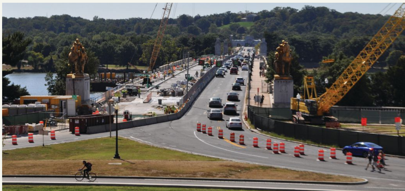
Two major construction stages temporarily reduced the six 10-ft-wide travel lanes to three 9-ft-wide lanes with a reversible center lane, allowing for closure of half of the bridge while the other half remained open. One of the two 14-ft-wide shared-use paths remained in service at all times. Photo: AECOM.
