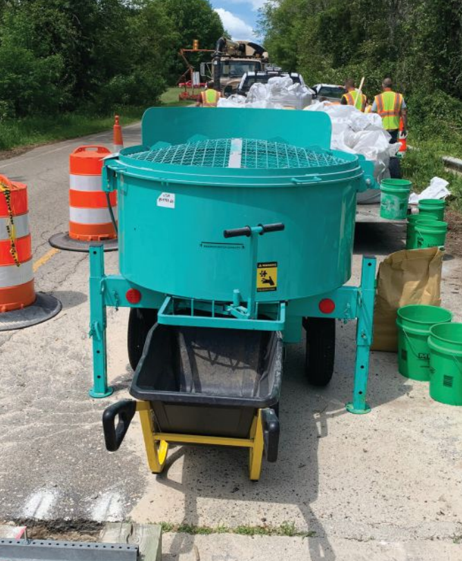
The mixer used by Clare County Road Commission staff to batch the open-recipe ultra-high-performance concrete in the field.
