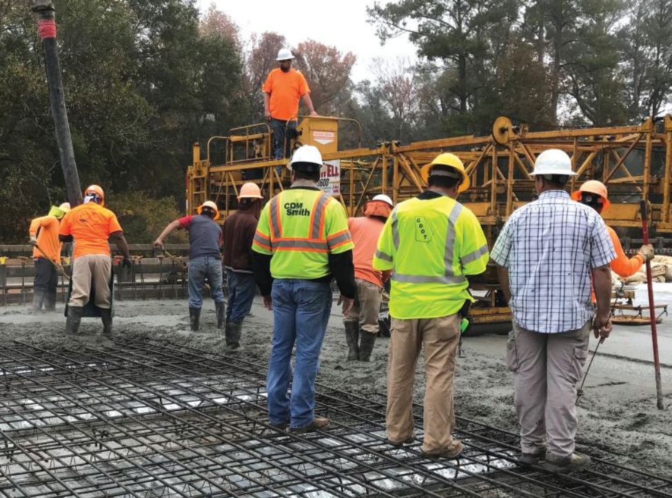
CDM Smith field personnel inspect the placement of concrete for a bridge deck.
