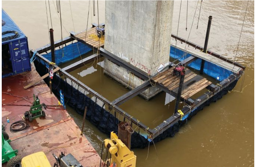
The North Carolina Department of Transportation approved the fabric concrete forming system using multiple layers of reinforced proprietary geotextile fabric developed by TrapBag Barrier Systems for the repair of a footing for the Lake Tillery Bridge rehabilitation project. All Photos: PCL Construction.
