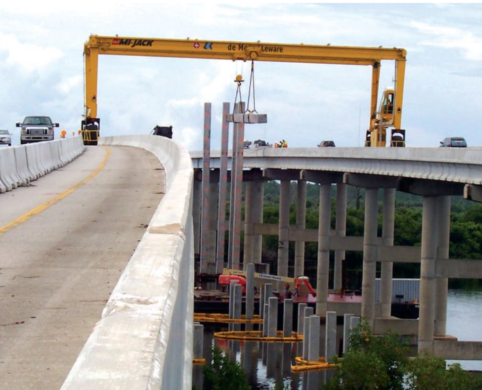
Figure 3. For the widening of Interstate 75 in Fort Myers, Fla., a gantry or straddle crane was the only solution. RTGs with clear spans of 84 ft cleared the median gap between the existing twin-span bridges. Two gantry cranes controlled by GPS, each having one set of tires on the west span and the other on the east span, minimized lane closures and lessened environmental encroachments.
