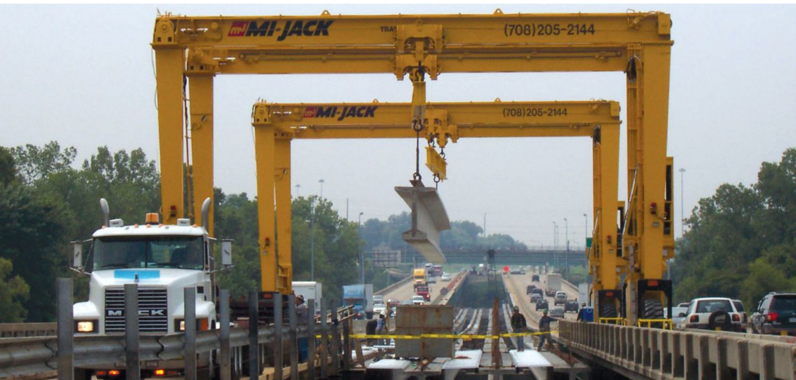
Figure 1. With the ability to straddle the gap between the existing structures, a rubber-tired gantry crane allowed work to progress on the Interstate 65 bridge over the Alabama River without lane closures. It also eliminated the need to transport cranes to other areas of the project. All Photos: Mi-Jack Products.
