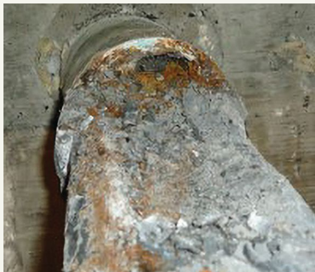
Figure 3. Corrosion of an external post-tensioned tendon at a location of soft, moist grout. Photo: Structural Technologies.
