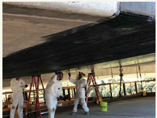
Figure 6. Carbon-fiber-reinforced polymer (CFRP) being installed to strengthen a concrete segmental bridge. Proper design, detailing, and installation is required for a CFRP strengthening system. Photo: Structural Technologies.
