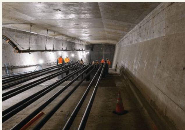
Figure 7. External post-tensioning tendons being installed to strengthen an existing concrete segmental bridge. Photo: Seattle Department of Transportation.
