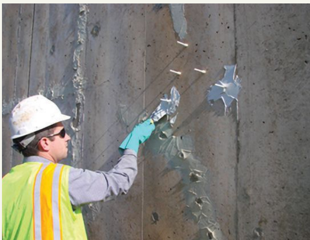
Figure 5. A cracked concrete element being prepared for repair with epoxy injection by installing grout ports and sealing the surface. Photo: Structural Technologies.
