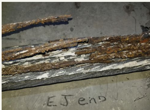
Figure 2. Corrosion of individual post-tensioning strands in an external tendon at a location where the duct was not completely grouted, leaving strands unprotected. Photo: Structural Technologies.
