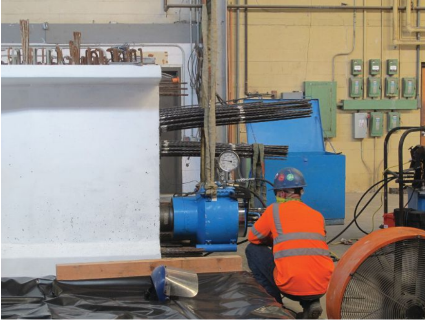
Stressing strands in a post-tensioning tendon for a demonstration specimen at the Ferguson Structural Engineering Laboratory (FSEL). Concrete Bridge Engineering Institute (CBEI) courses will include full-scale specimens for hands-on demonstrations of post-tensioning operations, including stressing. Photo: CBEI/FSEL.
