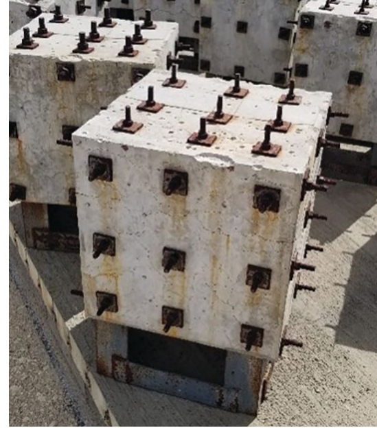
Concrete blocks that will be used in the Concrete Materials for Bridges Program. The blocks have different confinement and reinforcement details and show the effects of alkali-silica reaction. Photo: Concrete Bridge Engineering Institute.
