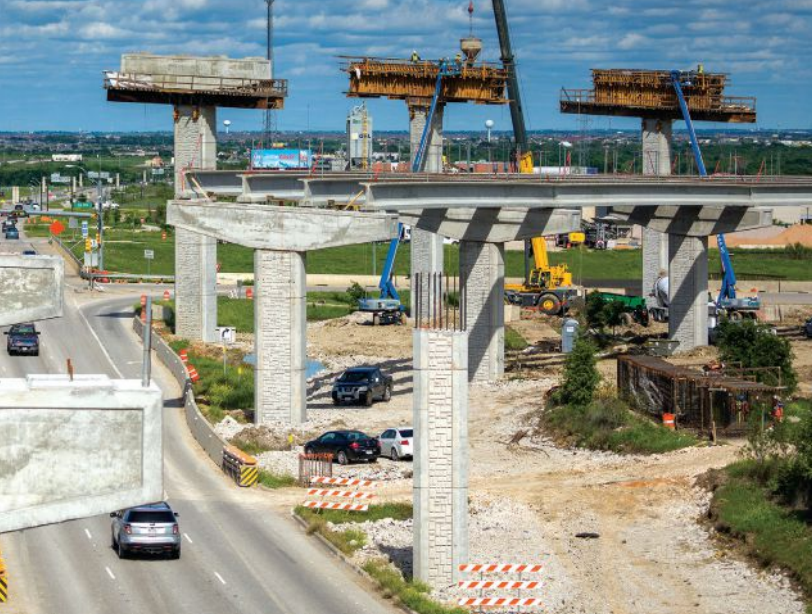
Crews simultaneously constructed piers for three new flyovers at the intersection of 290 Toll and State Highway 130.
