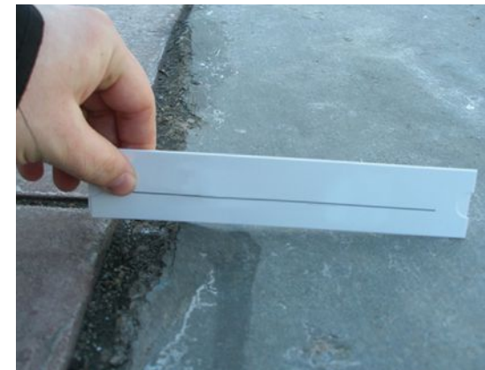
Figure 2. A concrete joint in the early stages of joint deterioration. A straight edge is used to show the expansion in the concrete near the joint caused by calcium oxychloride formation.
