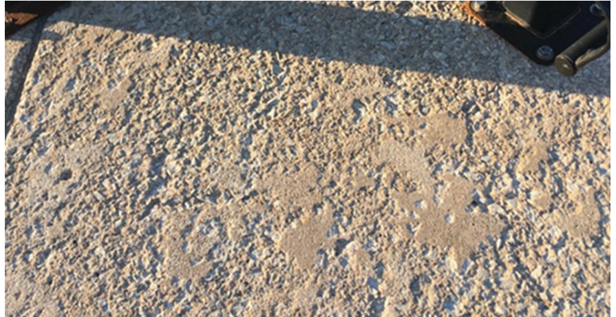
Figure 1. Concrete surface with severe salt scaling caused by use of deicers. All Figures and Photos: Kyle A. Riding.
