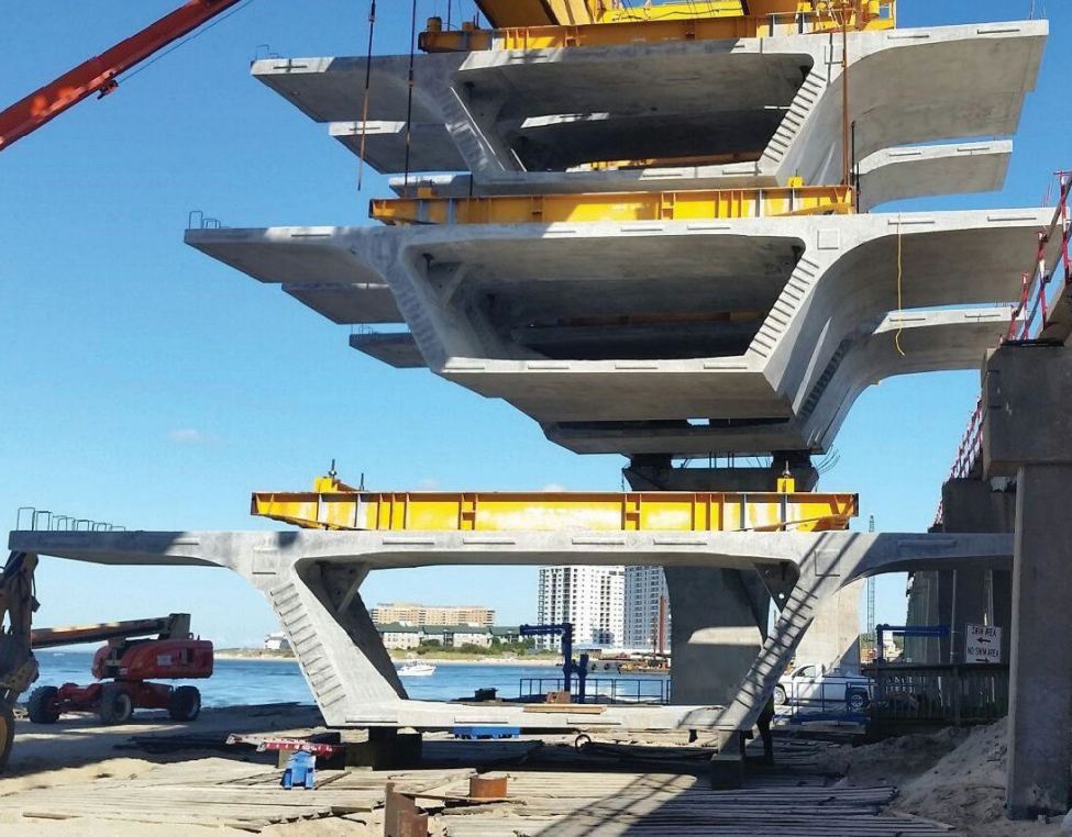
Precast concrete box-girder segments being erected for the Lesner Bridge project in Virginia Beach, Va. All Photos: RS&H Inc.
