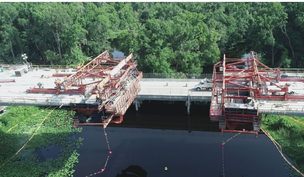
Construction of the main span cantilevers for the first of three cast-in-place segmental bridges for the Wekiva Parkway project in Sorrento, Fla. (see the Project article in the Fall 2020 issue of ASPIRE ®).
