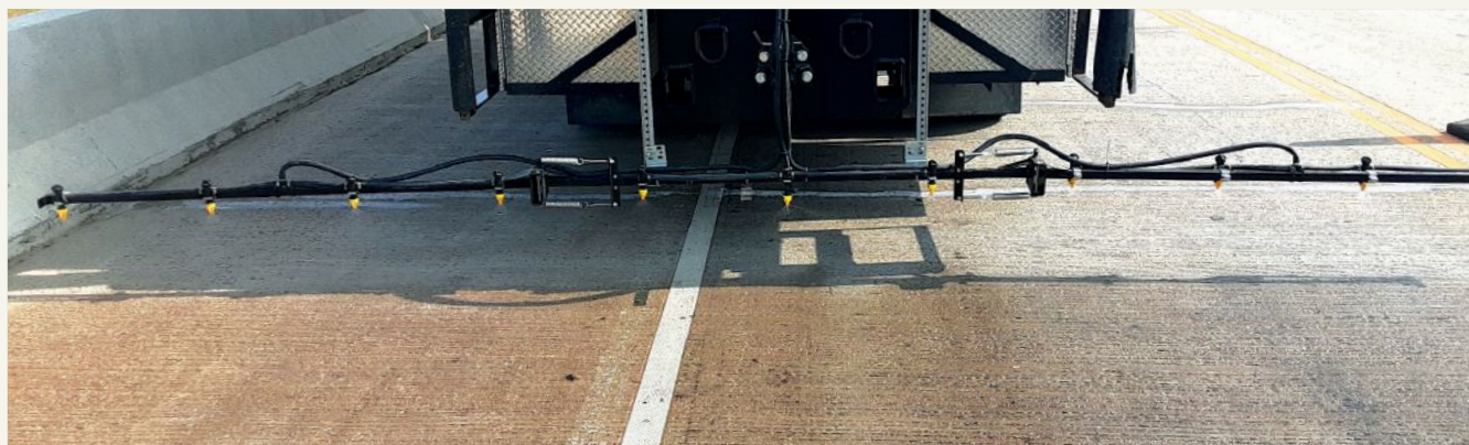
A spraying rig that can cover up to 100,000 ft 2 per hour applies modified silica gel to a bridge deck for the South Dakota Department of Transportation.
