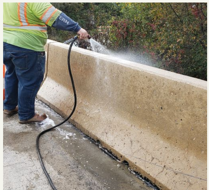
Water is applied to activate modified silica gel that was previously applied on a bridge barrier for a Delaware Department of Transportation project.
