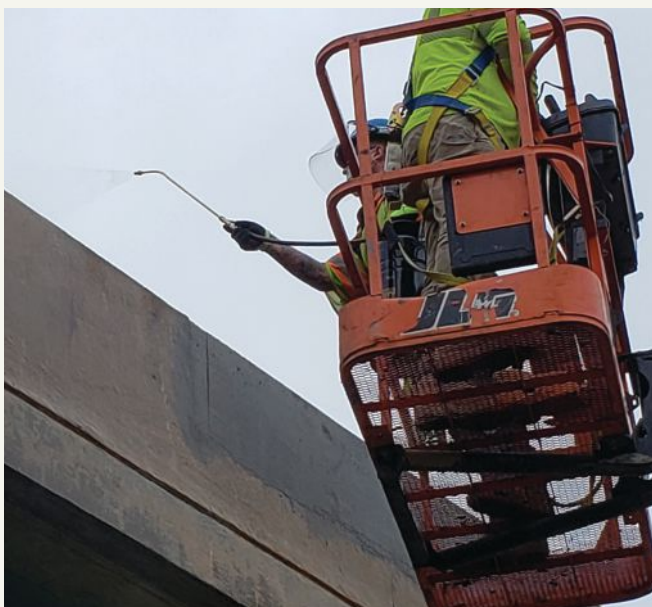
Spray application of modified silica gel on a bridge barrier for a Delaware Department of Transportation project. All photos: Alchemco.
