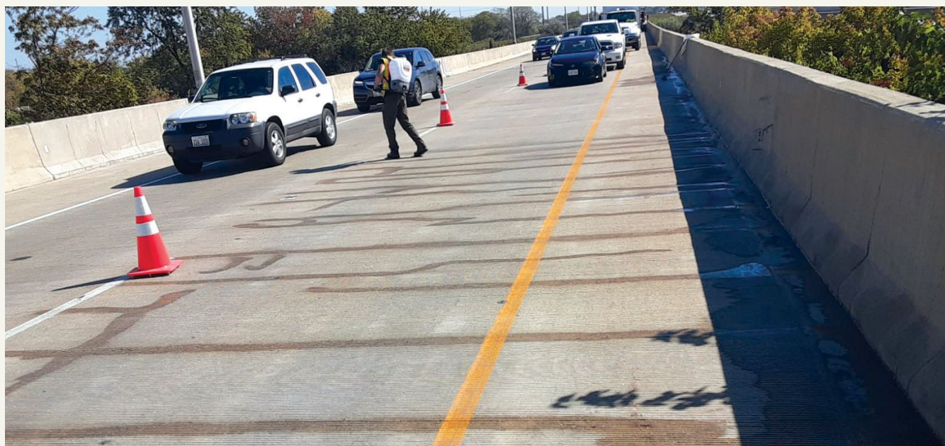
Modified silica gel is being applied to seal individual cracks in a bridge deck for the Illinois Department of Transportation.
