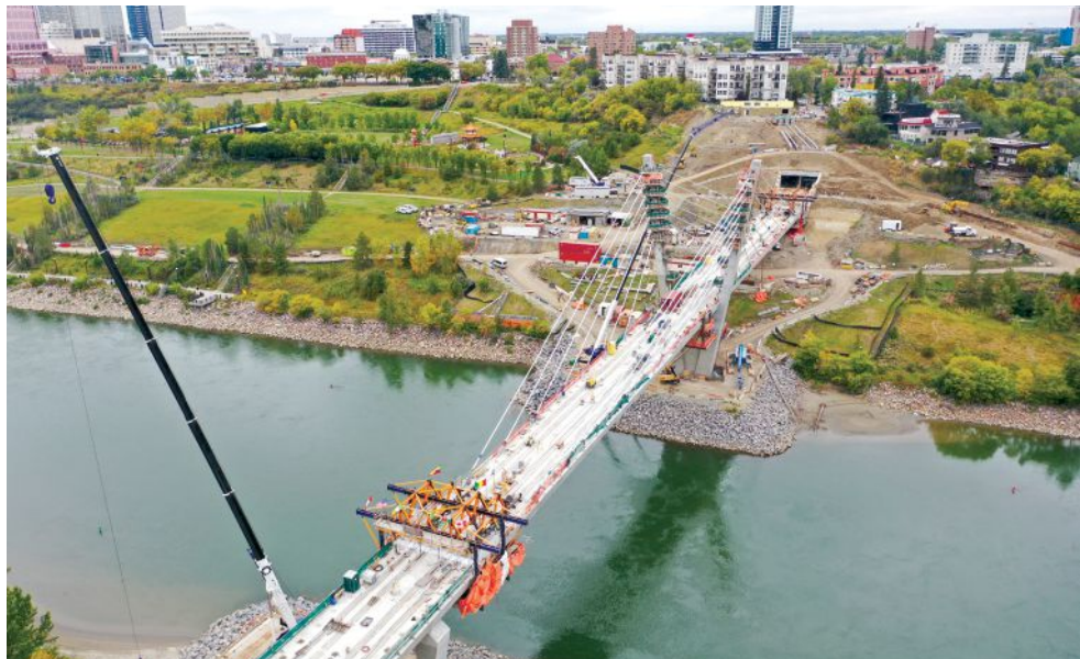
Tawatinâ Bridge is a new 853-ft-long extradosed light rail and pedestrian bridge over the North Saskatchewan River in Edmonton, Alberta, Canada. The structure is being constructed as a cast-in-place concrete, balanced-cantilever bridge using two moveable form travelers and is part of the 27-km Edmonton Valley Line light rail transit design-build project. Photo: TransEd Partners.
