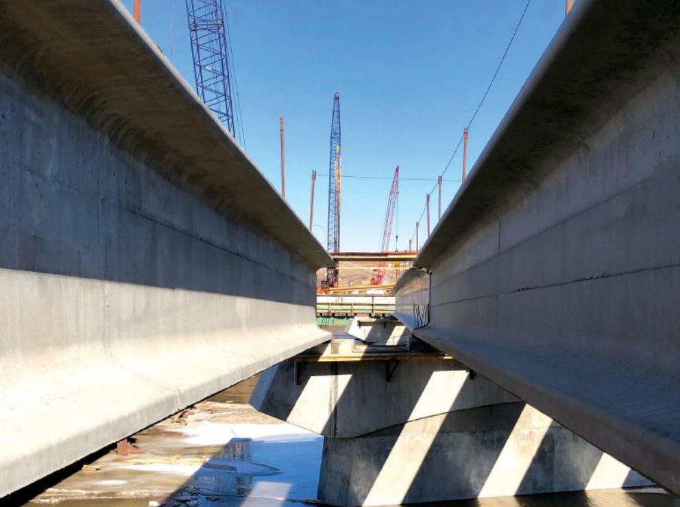
Looking along the NU1800 precast, prestressed concrete girders toward one of the permanent bridge piers.
