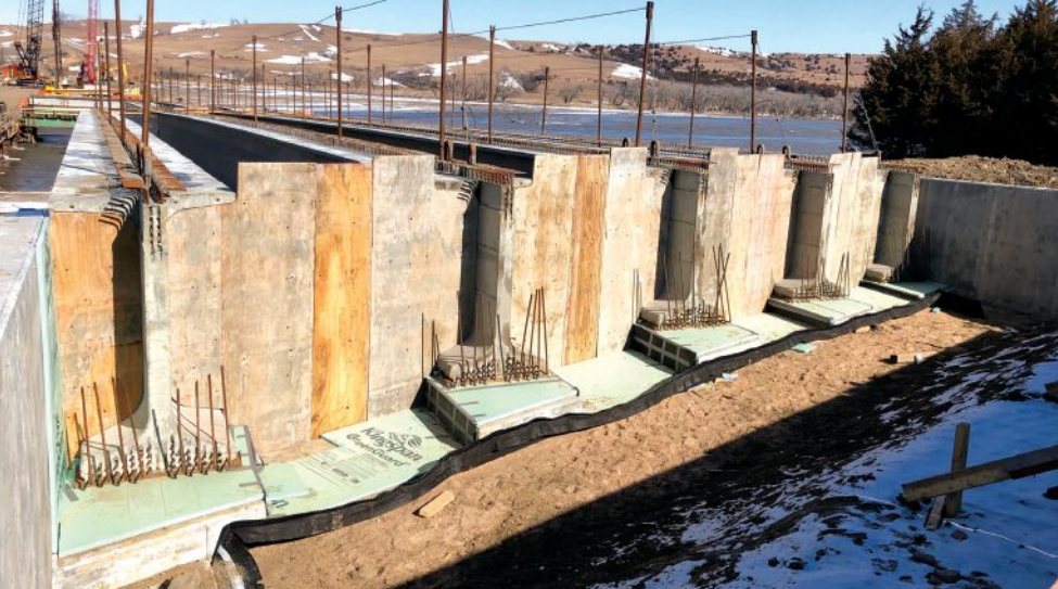
A view of the skewed ends of the NU1800 prestressed concrete girders at an abutment. This photo was taken before the semi-integral abutment turnout placement and before the deck forming and concrete placement. This bridge featured a jointless deck system across the length of the structure. Expansion joints were placed at the end of the approach slabs, which were founded on pile-supported grade beams placed 20 ft beyond the abutments.
