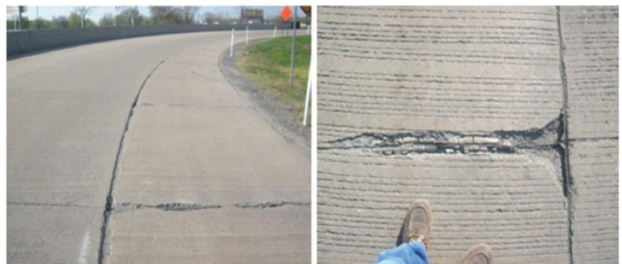
Figure 1. Example of concrete pavement joint damage showing cracking parallel to the joint and spalling and cracking at the joint. Photos: Jason Weiss.
