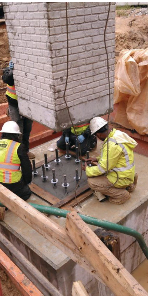
After a dry-fit test of the column on the footing to ensure proper fit of dowel bars and couplers, the grout bed was prepared for final setting of column. Two rows of ports for grouting couplers are visible at the base of column.
