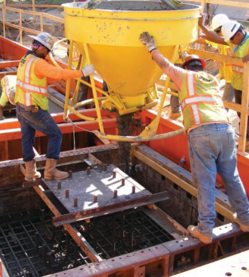
A steel template based on the bar-coupler locations in the precast concrete columns was used to position the no. 11 dowel bars while placing concrete in the footings.
