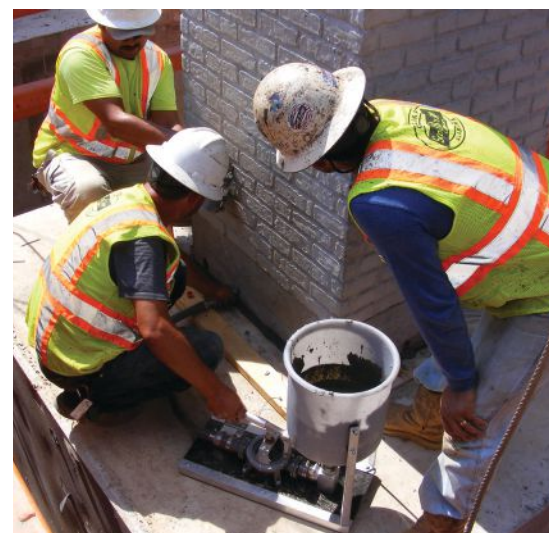
Grout was pumped into the couplers according to manufacturer's instructions, but some locations required a modified approach to address challenges encountered during construction.
