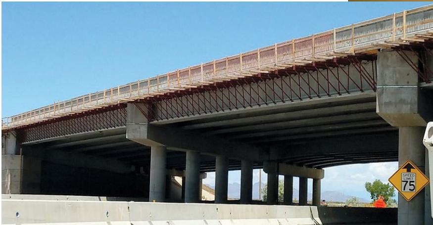
Views comparing the Tooele Interchange at Lake Point Bridge model and the structure during construction.
