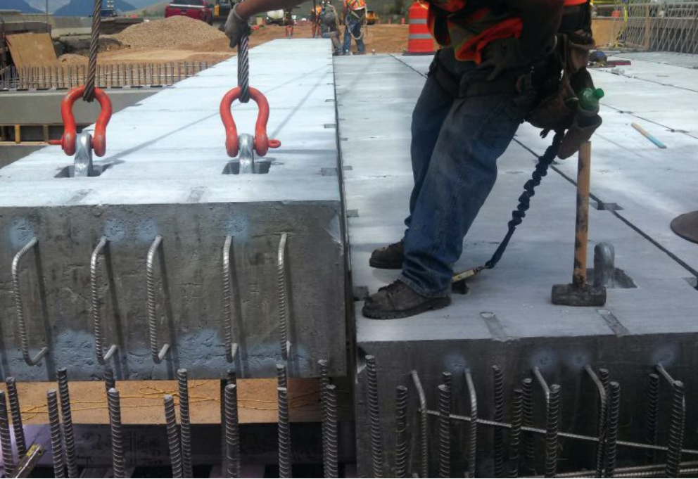
Placement of a voided-slab girder on the precast concrete diaphragm for the Interstate 84 Bridge over Echo Frontage Road. All reinforcement in the bridge is stainless steel.
