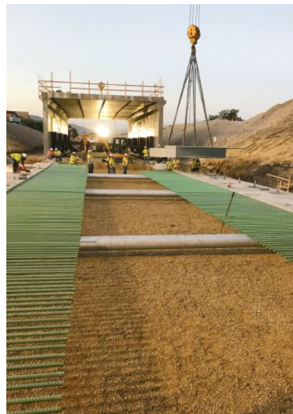
Precast concrete footing section being set for the Interstate 15 Northbound/10600 South Interchange three-sided box structure. In the background is the box structure where it was staged before the slide. After the slide, the section between the parallel precast concrete footings was cast in place to complete the bottom slab of the structure's foundation.
