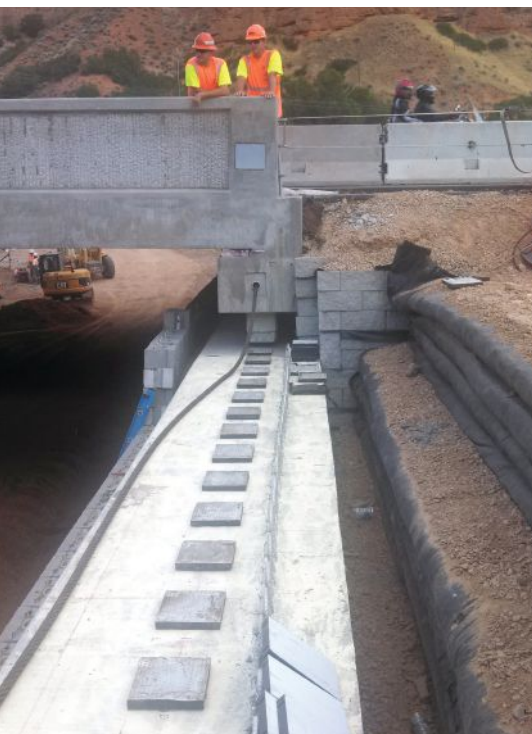
Neoprene bearing pads on the bearing sill of the Interstate 84 Bridge over Echo Frontage Road before the slide. The reinforced layers of fill in the GRS-IBS abutment are visible on the right.
