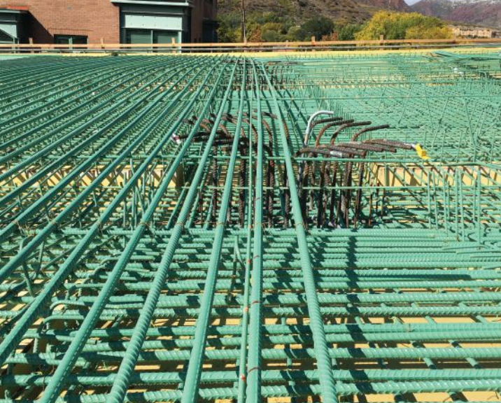
Epoxy-coated reinforcement was used in the slab. The reinforcement projecting into the slab from an integral column is visible.
