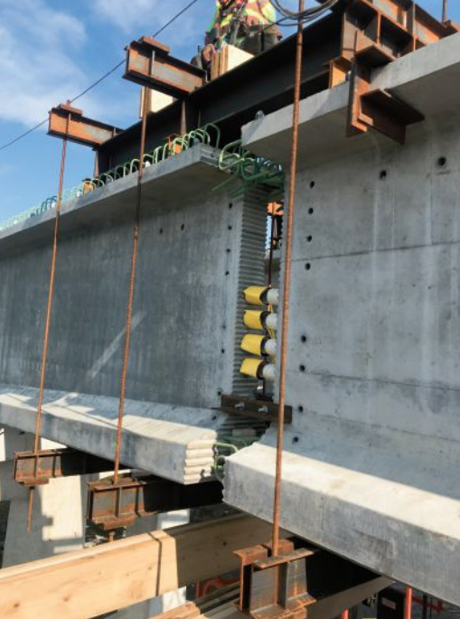
Girder splice with strongback support. The 1-ft-wide gap between girder segments for post-tensioning duct splicing was later filled with 9000-psi cast-in-place concrete, which was placed simultaneously with the diaphragms. Photo: AECOM.
