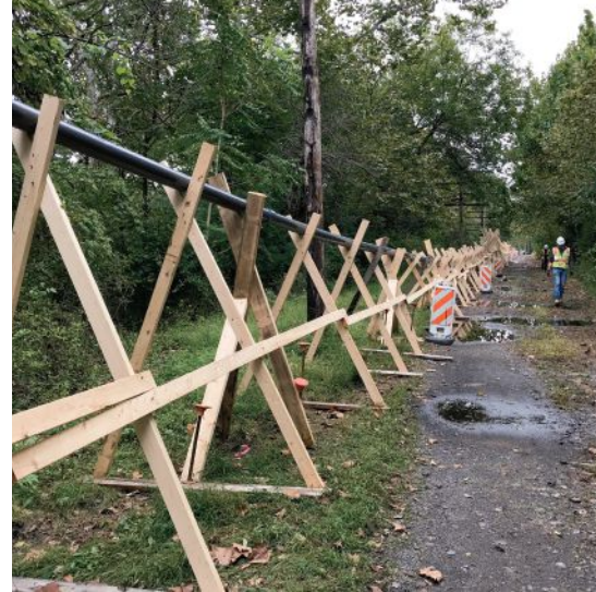
The contractor was required to provide a mock-up of a single 540-ft-long tendon duct to demonstrate the ability to completely encapsulate the strands in the tendon with grout from end to end. Clear plastic duct was used at critical points along the profile for inspection purposes. Photo: AECOM.
