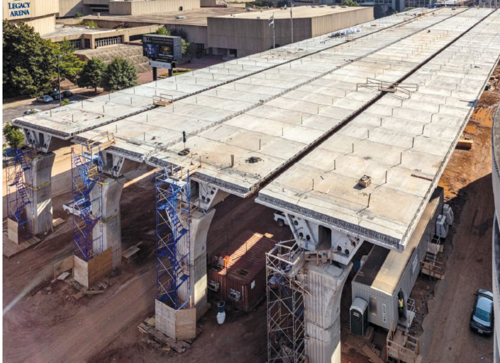
A typical span after erection of the four lines of box-girder segments. A longitudinal closure pour about 3 ft 6 in. in width was used to join the segments for each of the two bridges. The completed eastbound and westbound structures are separated by a 6 in. gap. Photo: Volkert Inc.
