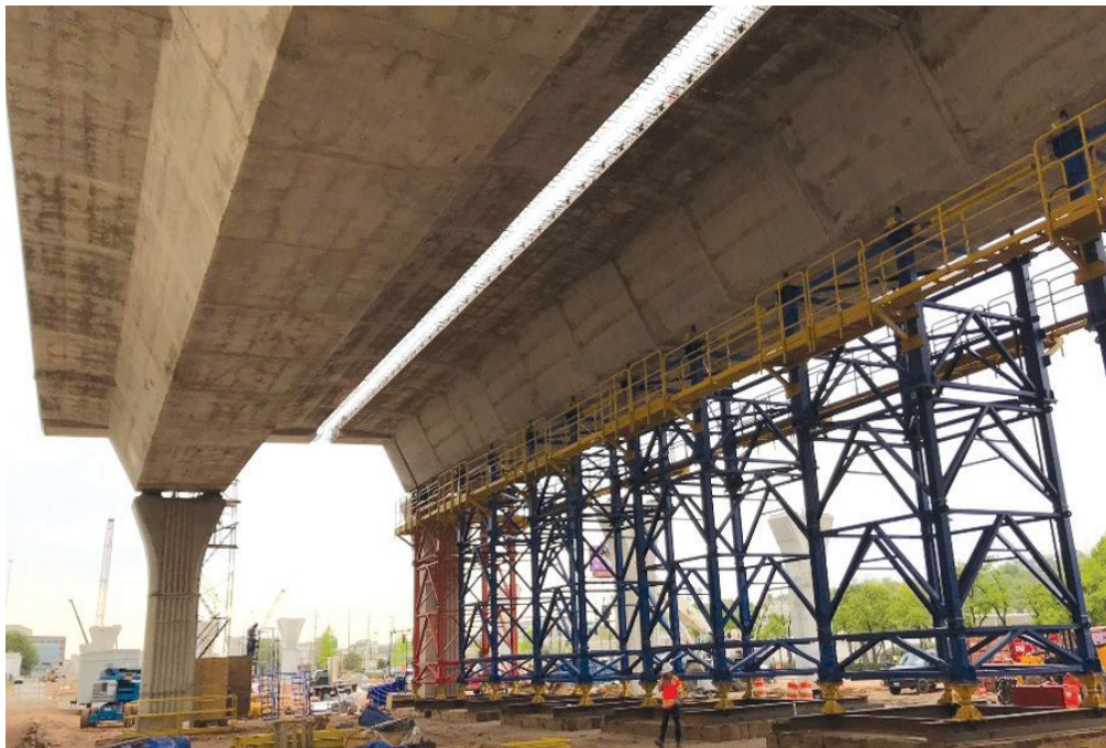
Falsework towers were used to support segments during erection. Photo: Volkert Inc.
