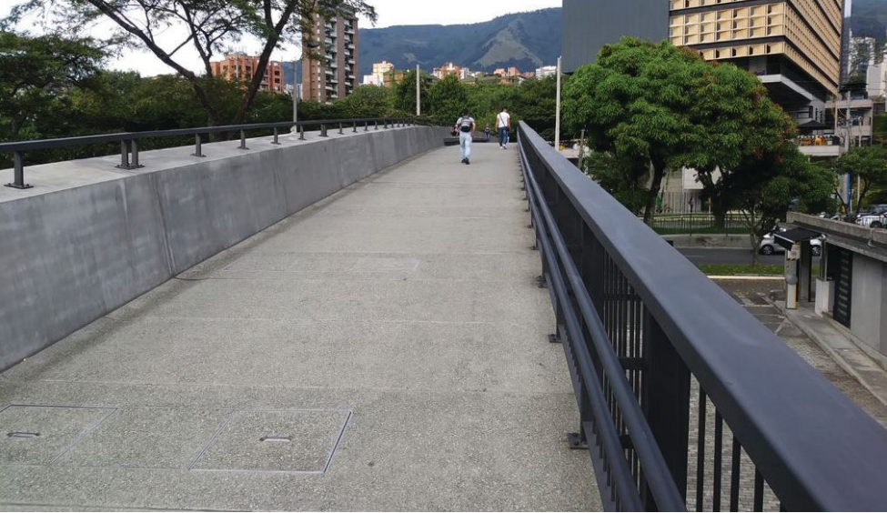
This segmental, post-tensioned pedestrian bridge in Medellín, constructed in 2017, is the first ultra-high-performance concrete bridge in Colombia.
