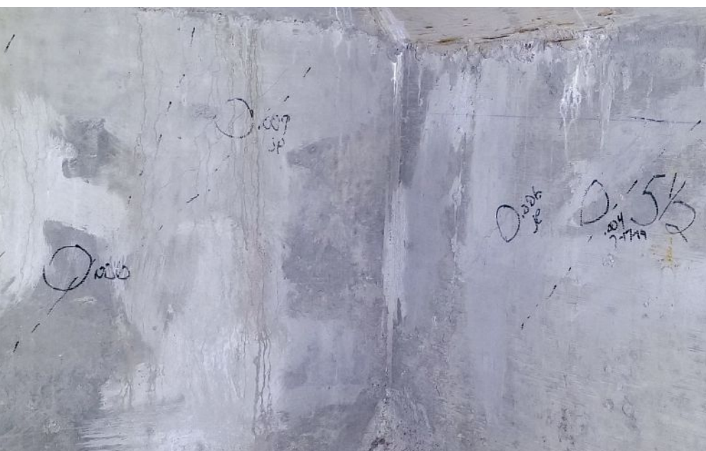
Figure 4. Diagonal cracking (dashed lines) noted during inspection of an integral cap beam of the Lake Avenue Bridge. Cap beam is on the left, and girder web is on the right. Photo: Minnesota Department of Transportation.
