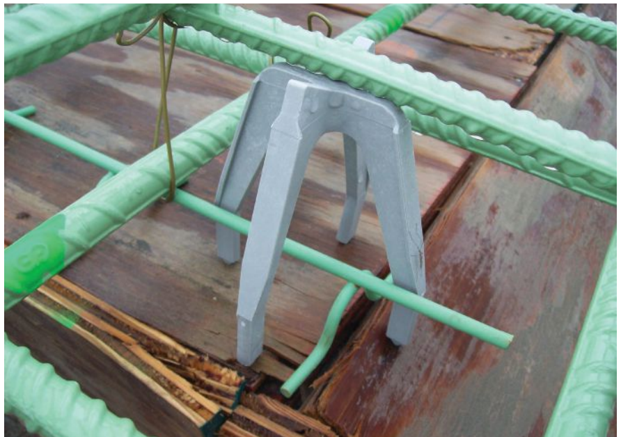
Epoxy-coated reinforcing steel placed on epoxy-coated wire and plastic bar supports. All Photos: EIG.
