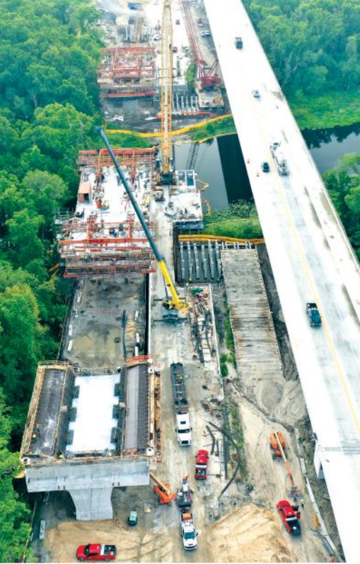
Aerial view of segmental bridge construction in several stages: The completed first bridge (on the right) is open to traffic; construction on the outer bridge (on the left) is progressing from two main piers; and foundation construction has begun on the center bridge after demolition of previous bridge. Photo: Superior Construction Company Southeast.
